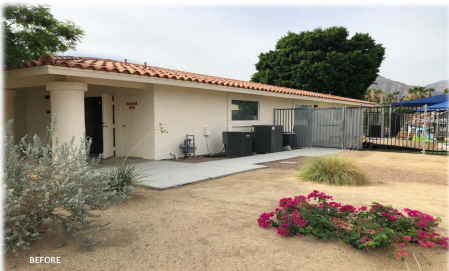
YMCA BACKUP GENERATOR
