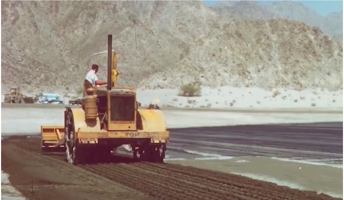
Figure 9. Lake Cahuilla Reservoir Under Construction 1969 (Courtesy of the Coachella Valley Water District https://cvwatercounts.com/watch-film-shows-creation-of-lake-cahuilla-in-1969/ )
